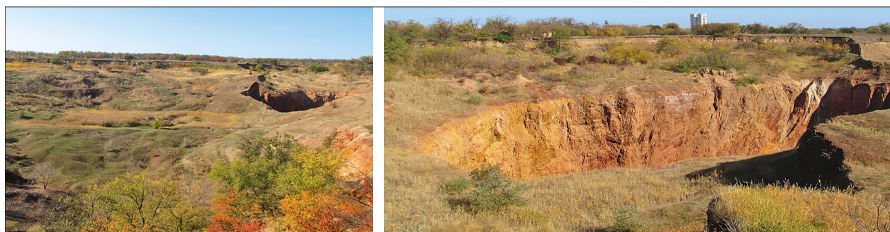
Figure 13. Sinkhole No. 4 (photo by Dmitry Antonov, 2015)
