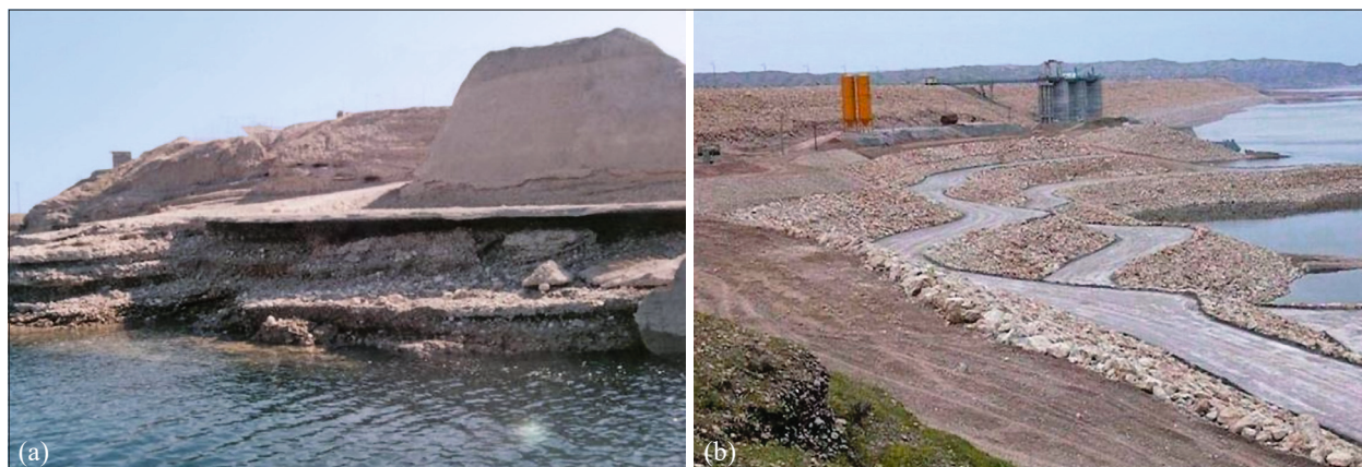
Figure 3: (a) shoreline erosion caused by wave action; (b) soil-cement and supplementary embankment earth fill
